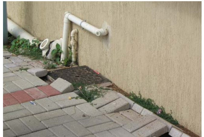
Fig 8. Damage to wet services as a result of leaking paving
