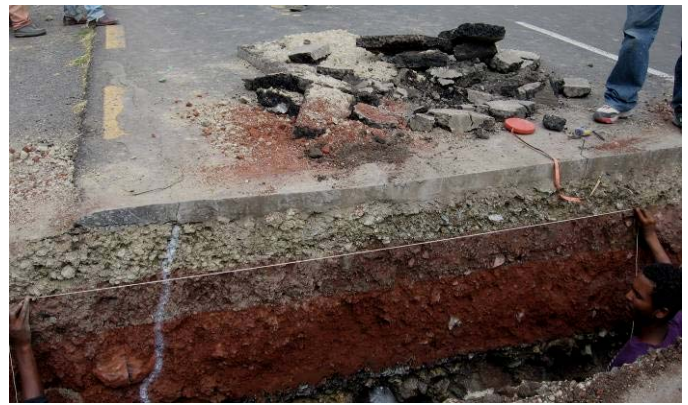
Fig. 4. Crack propagation in outer wheel track
