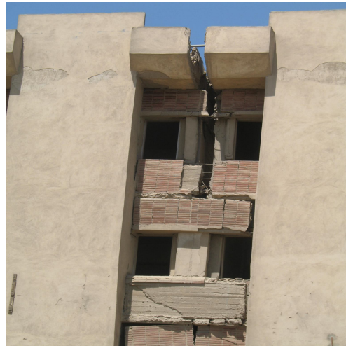
Photo 2 Break of beam and column near expansion joint.
