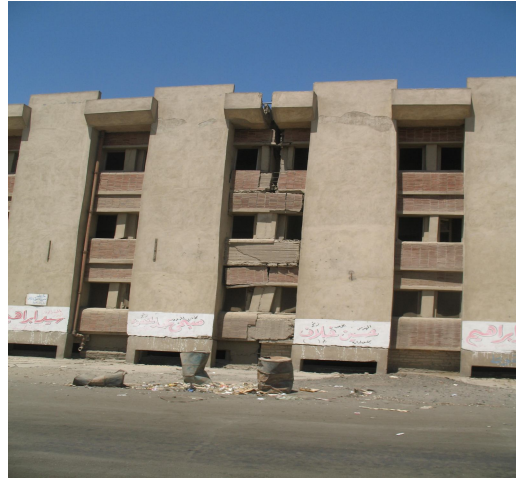
Photo 1 An increase of expansion joint
