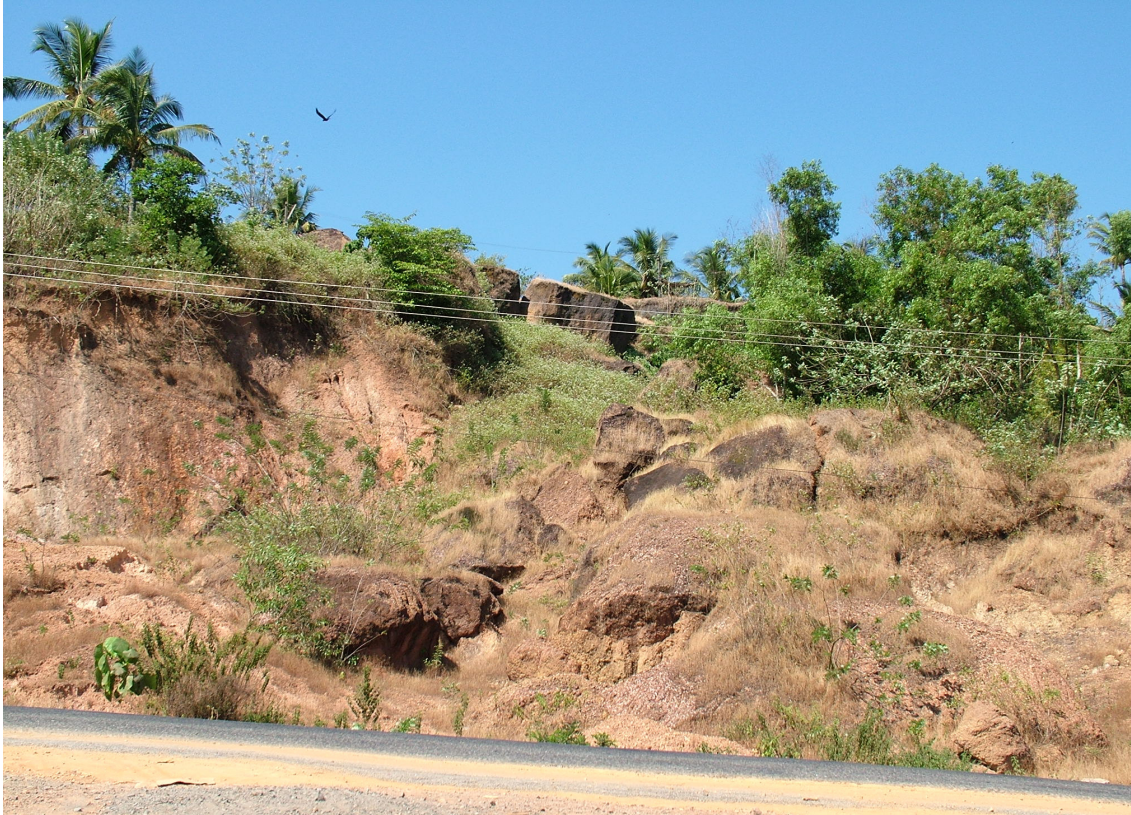
Fig5: View of Kethikal land slide from the road level.
