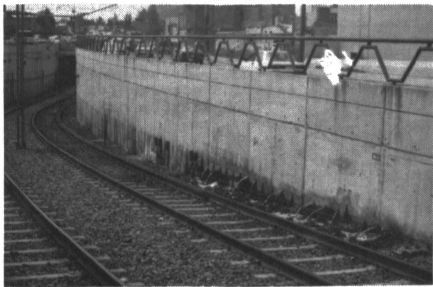
Fig. 9 Water Inflows Into the Access Ramp
