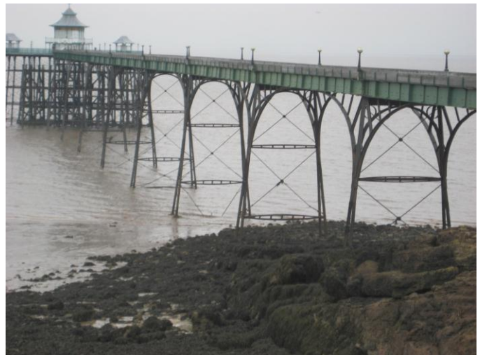
Fig. 8. 2011 Photos of the Piers at Weston-Super-Mare (upper) and Clevedon (lower).
