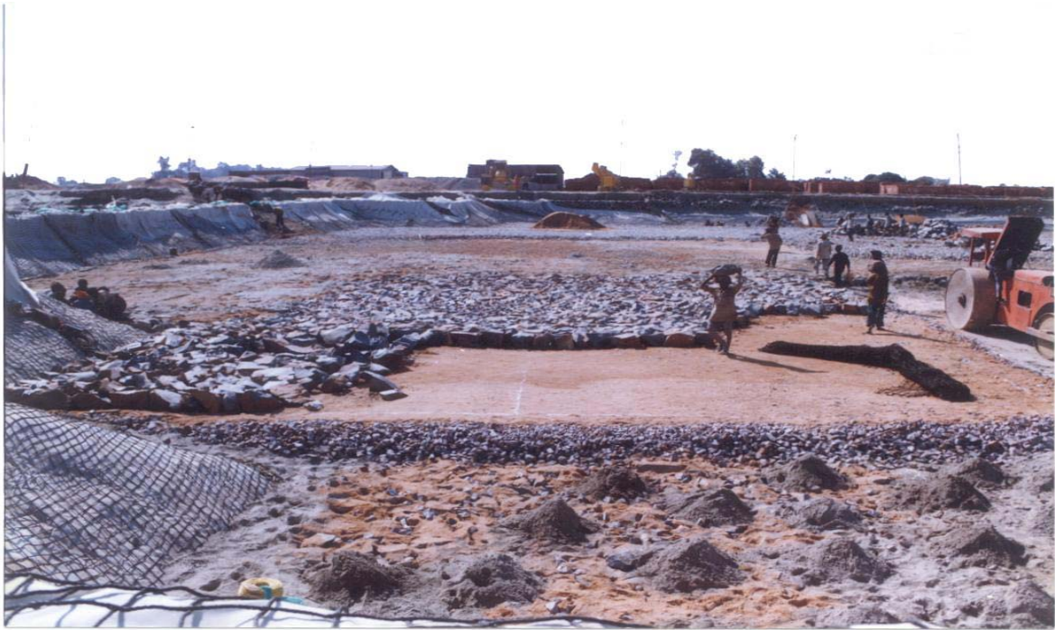
Fig.6(a). Sequential construction of the foundation system shown in fig 5 in a typical cross section
