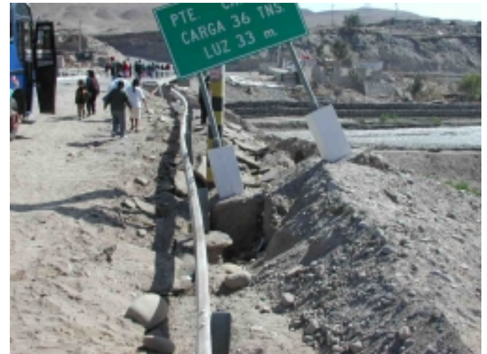
Fig. 9. Liquefaction-related damage at the Locumba bridge site.
