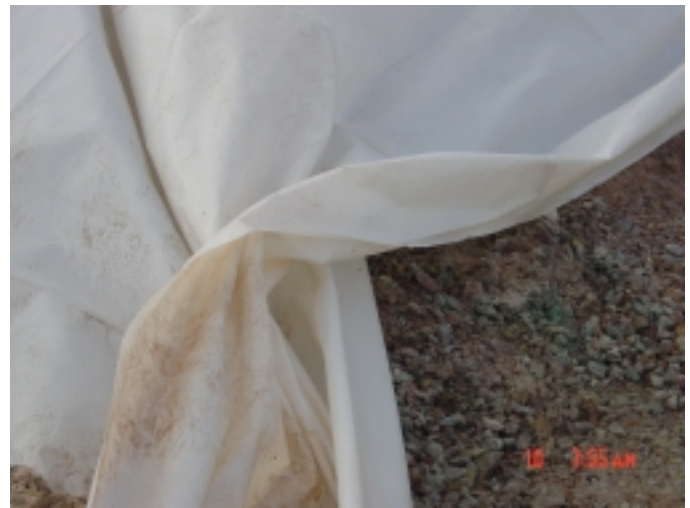
Fig. 6. . Ore at failed heap leach pad at mine.
