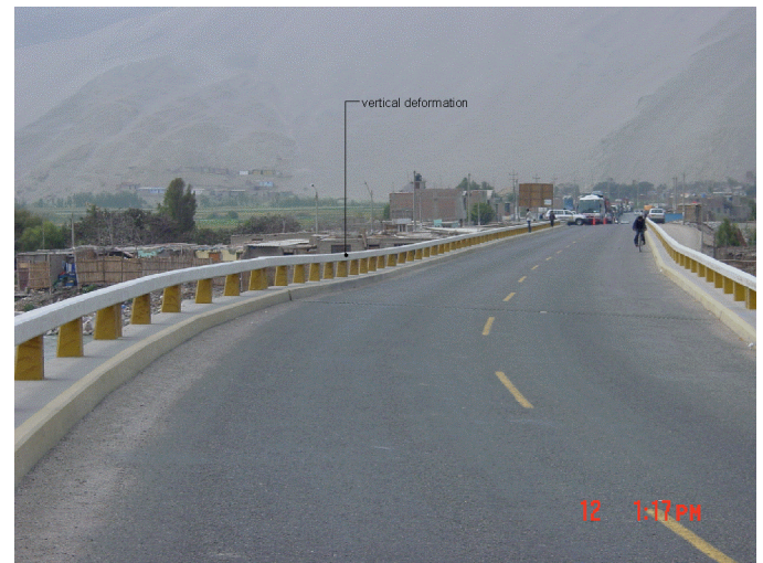
Fig. 12 Vertical deformation in the Ocoña Bridge probably resulted from liquefaction-induced foundation movements.
