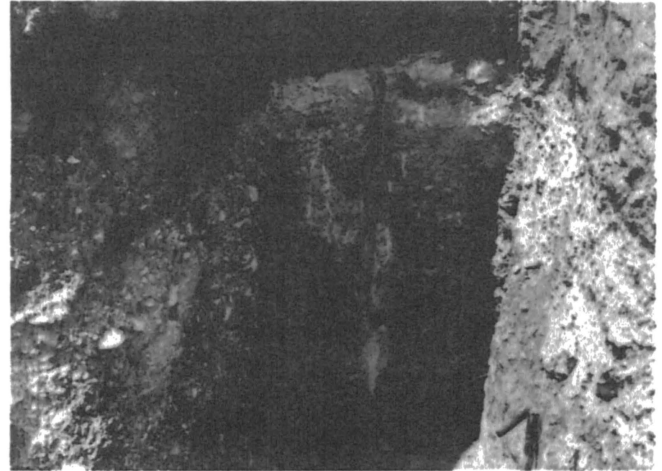
Fig. 5 Defects in North Cut-off Wall
