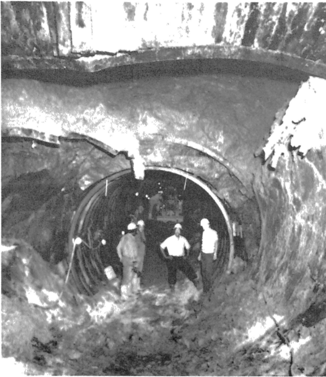
Fig. 6. Corridor Interceptor Tunnel Distress
