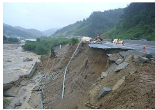
Pic.1 Destroyed embankment
