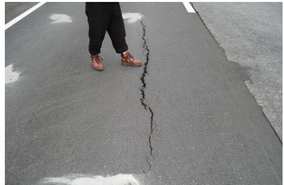
Pic.7 Cracks of the westbound lane pavement
