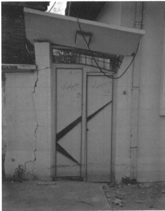
Fig. 7. Liquefaction-Induced Differential Settlement Between a House and an Adjacent Wall in Astaneh-Ashrafieh
