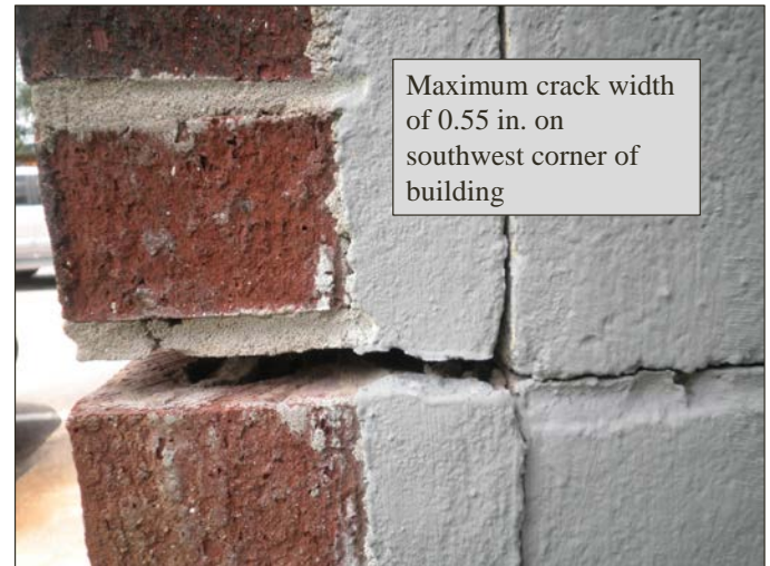
Fig. 4. A crack 0.55 in. wide observed on the southwest corner of the building.
