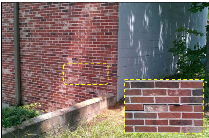
Fig. 3. Observed Cracks on the front brick façade of the building.
