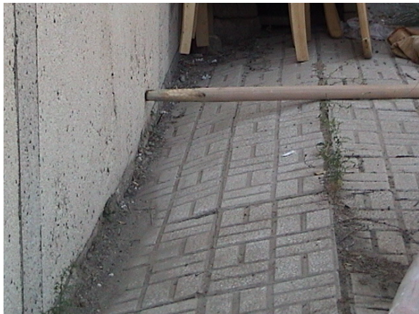
Fig. 1 Damages to flooring due to the swelling of gypsum soils
