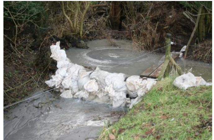
Figure 5: Sand boil surround by sand bags (Picture by Laurens Pompe, Waterschap Rivierenland)
