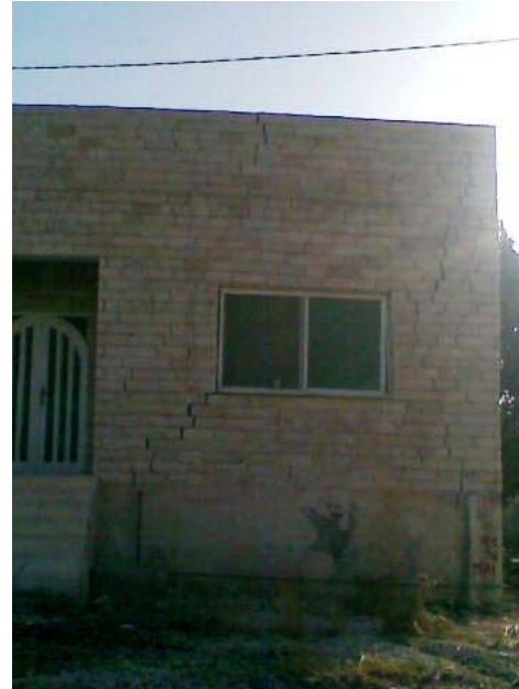
Fig: 4 Damaged Building: diagonal and vertical cracks
