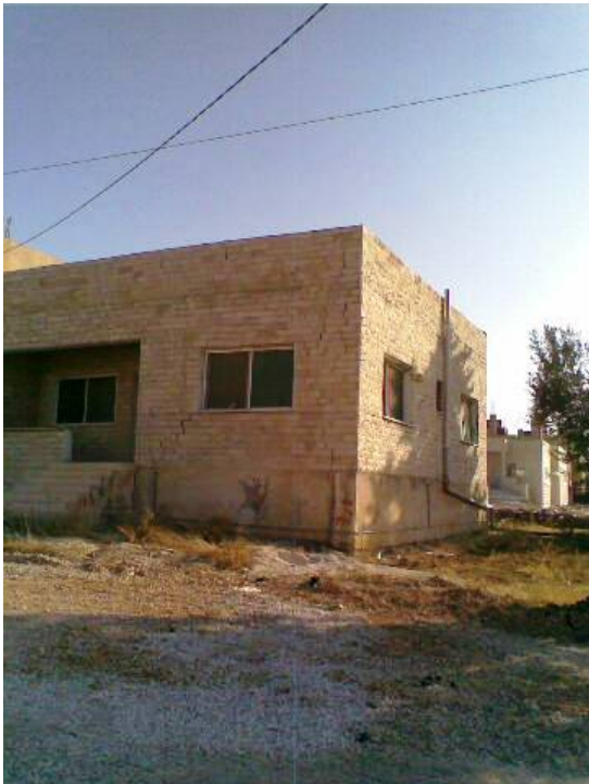
Fig: 3 Damaged Building: evacuated damaged portion
