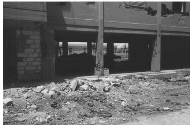
Fig. 2. Damages occurred on buildings.
