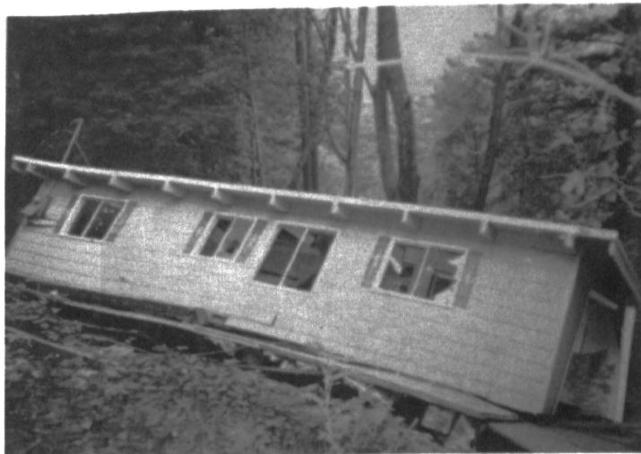
FIGURE 3 HOUSE THAT WAS NOT BOLTED DOWN WAS KNOCKED OFF IT'S FOUNDATION DURING THE LOMA PRIETA EARTHQUAKE
