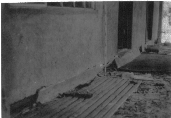
FIGURE 4 LATERAL SHIFTING OF THE FLOOR STRUCTURE OVER THE FOUNDATION CREATED BY A LACK OF BRACING OF THE CRIPPLE WALL
