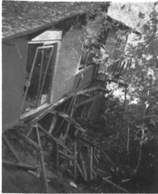
FIGURE 5 RACKING OF POST-AND-PIER FOUNDATION ON MOUNTAIN SIDE FROM SHAKING
