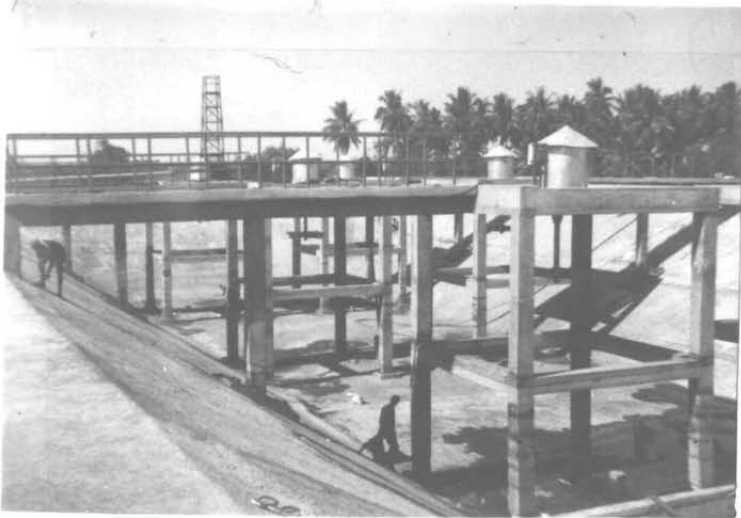
Fig. 2 Photograph of general view of aeration tank.
