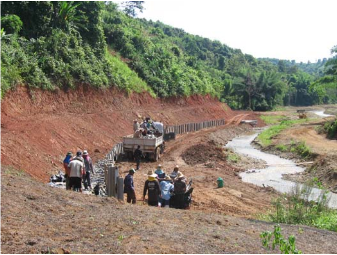
Fig. 8 A photograph showing the preparation of the reinforcement site at the base of the hill slope next to the stream channel.
