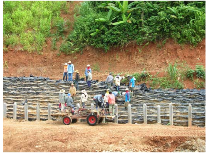
Fig. 9 A photograph showing the piling of soil bags as a part of the reinforcement of the slope at its base carried out by local people task force.
