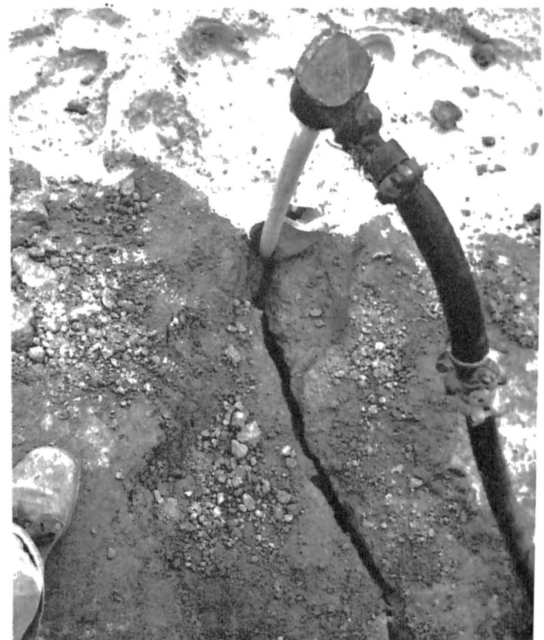
Fig. 11. View of a Crack in the Fill.
