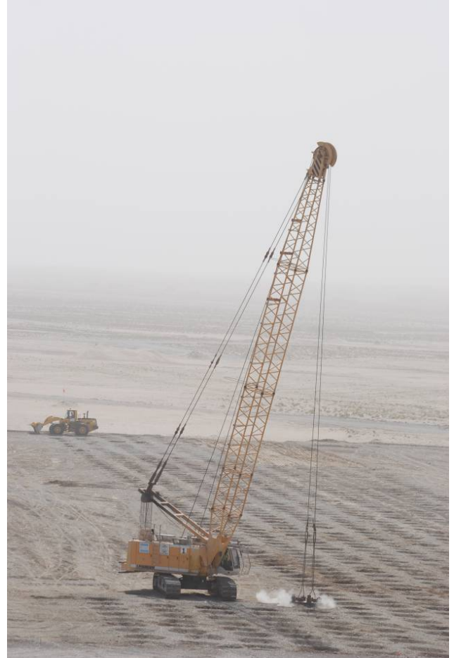
Photo 1. Typical configuration for Falling Weight Treatment, also known as Deep Dynamic Compaction - DDC.
