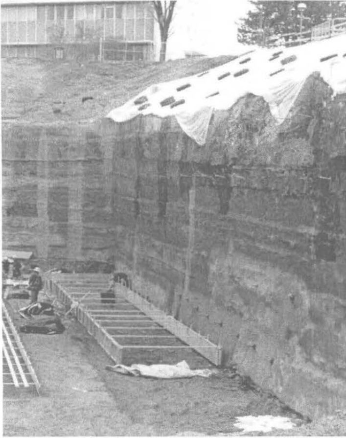
Figure 9: Photograph of soil-nail wall on east side of excavation of BYU library.
