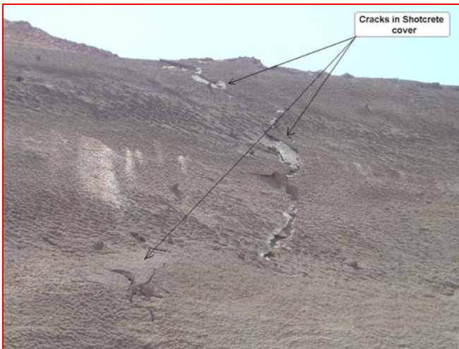
Fig. 9. local cracks that occurred in shotcrete cover
