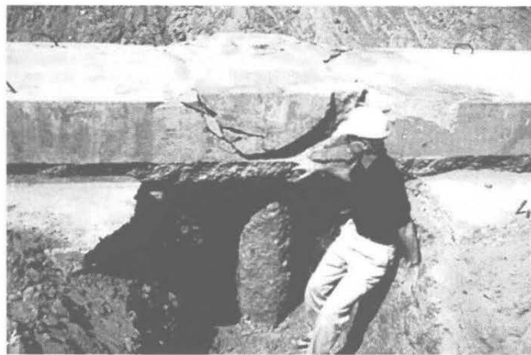
Fig. 3 Punching shear failure of Delta pile through pile cap.
