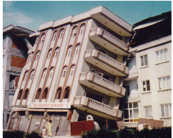
Fig.11. Liquefaction induced foundation failure in Adapazari during the Kocaeli earthquake
