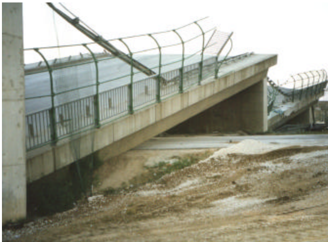
Fig.13. Unseating of bridge decks from piers of the Arifiye Bridge traversed by surface fault
