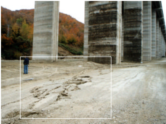
Fig.12. Piers of Trans-European-Motorway (TEM) traversed by surface fault rupture, Kaynasli, Düzce
