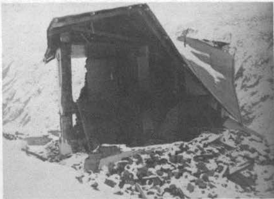
Fig. 16. Collapse of check post at Shalkar on India-Tibet road. Big boulder rolling down from hill slope caused collapse of the building.
