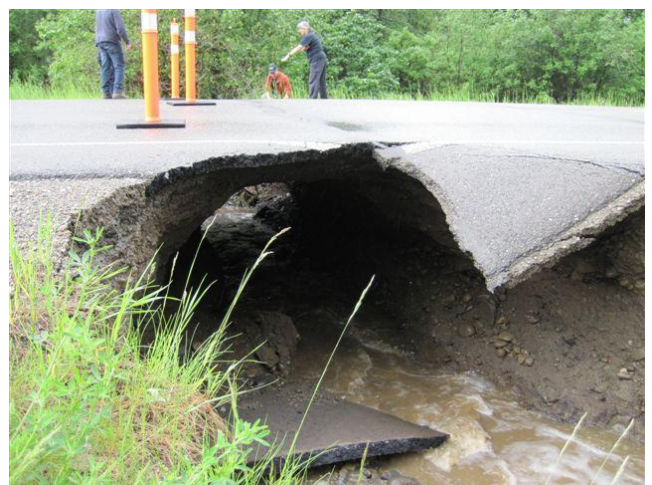
Fig. 8 Highway 97, Pinepass- Chetwynd – USA Flood Damage
