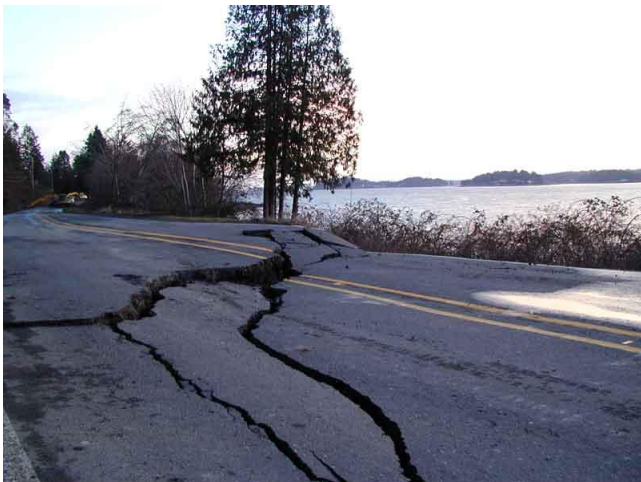
Fig. 10 Extensive road damage during 2011 Nisqually Earthquake in Washington
