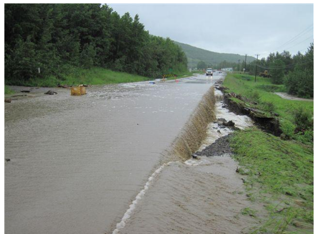
Fig. 7 Flooded Highway 97, Pinepass- Chetwynd – USA
