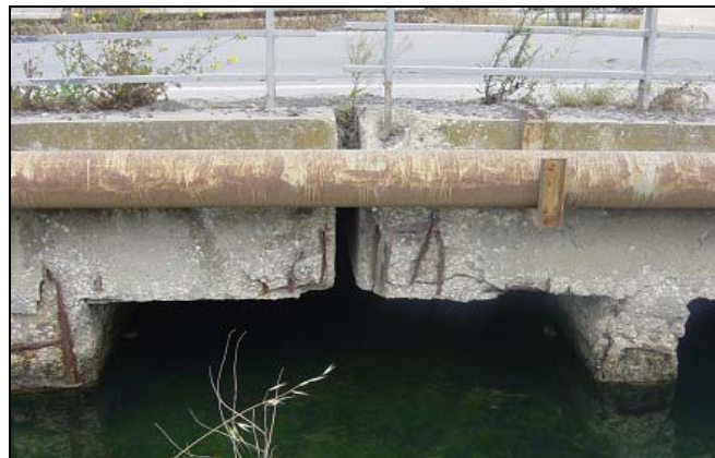
Photo 4. Rotation of piers
