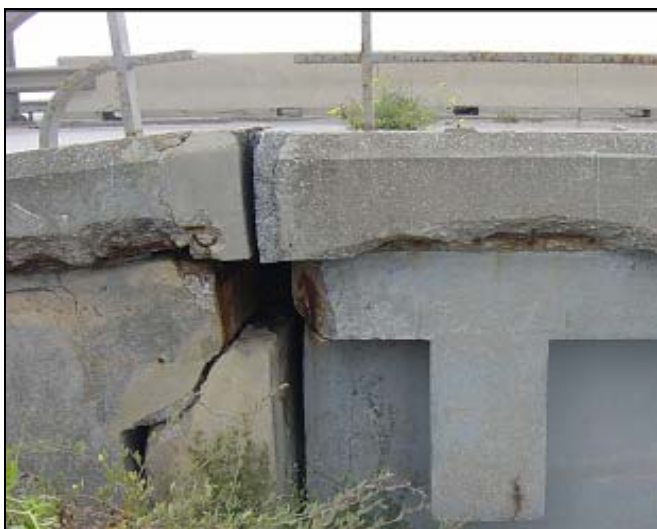
Photo 3. Rotation of approach slabs followed by structure damages.
