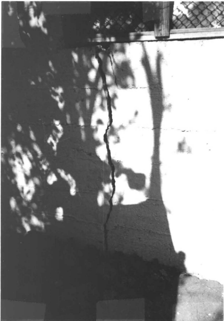
Photo 3. Damages registered at building No. 53
