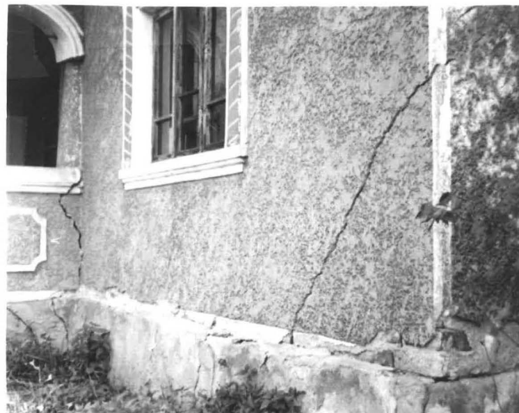
Photo 2. Damages registered at building No. 14
