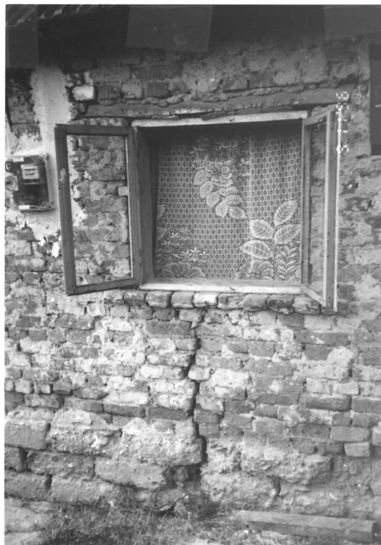
Photo 4. Construction defects at the building No.49
