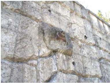
Fig. 9 (c) Cracks or flake off of the concrete blocks
