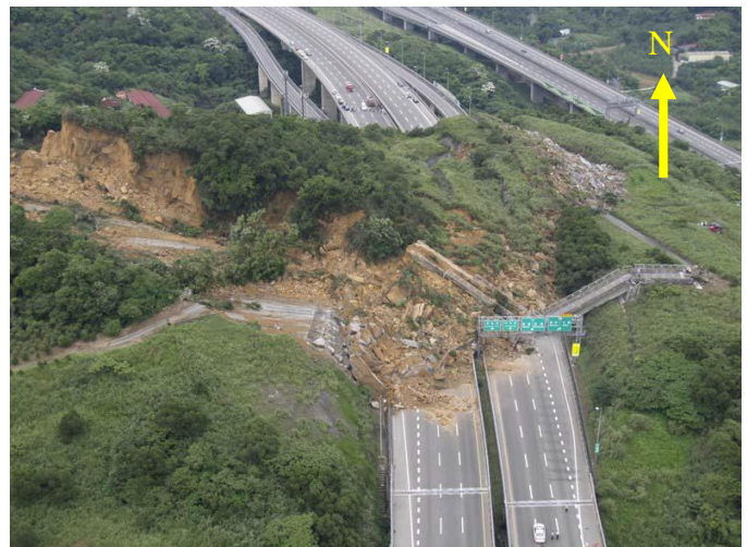
Fig.1 Photos of slope failure on Formosa Freeway in Taiwan
