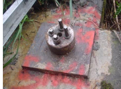
Fig. 10 (b) Tendons uneven shrink caused by angular bending Fig. 10 Tendons angular bending conditions
