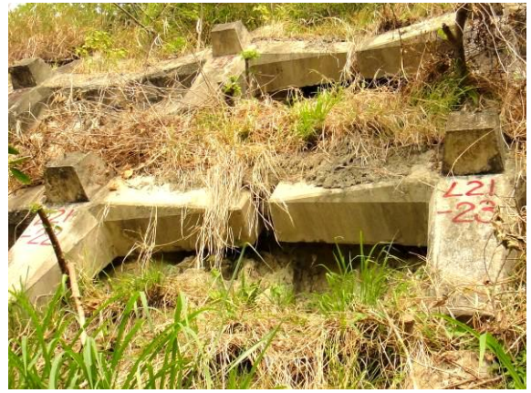
Fig. 12 (b) Topsoil hollowed Fig. 12 Prestressing lose conditions
