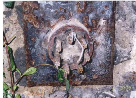
Fig. 11 (a) Anchor head corrosion
