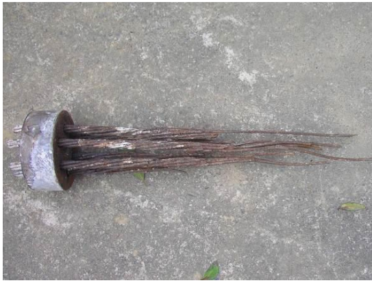
Fig. 11 (c) Corrosion and breaking of free length tendons
