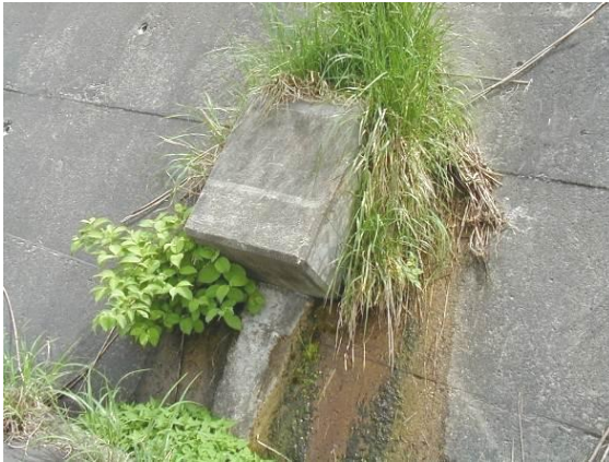
Fig. 11 (d) Efflorescence or groundwater seeping out Fig. 11 Anchor head corrosion and wedges slip and breaking of tendons
