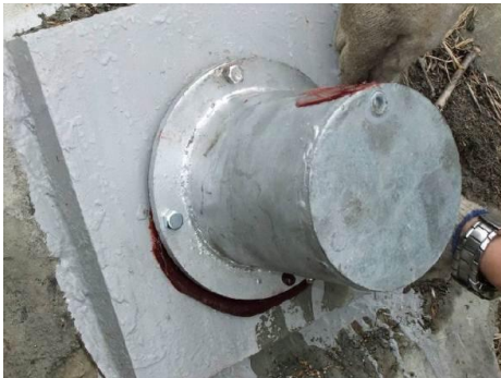
Fig. 16 (d) fixed galvanized cover with bolts Fig. 16 Construction process of corrosion-inhibiting cover
