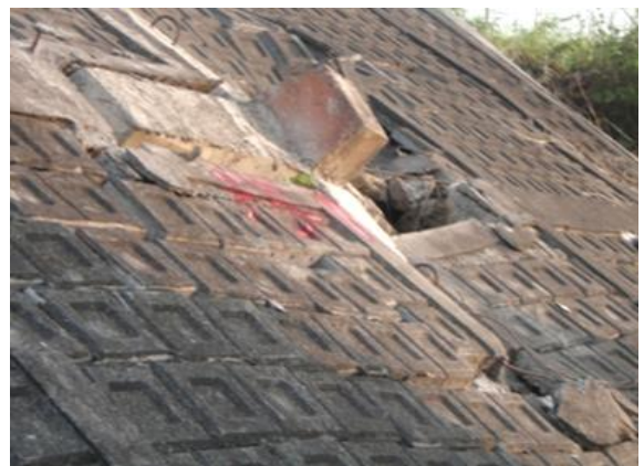
Fig. 13 (b) Anchor head sink Fig. 13 Failure conditions of anchor head
