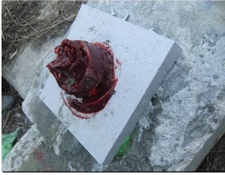
Fig. 16 (b) filled anchor head with corrosion-inhibiting compound
