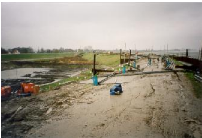
Fig. 8. Dyke failure due to uplift mechanism.
