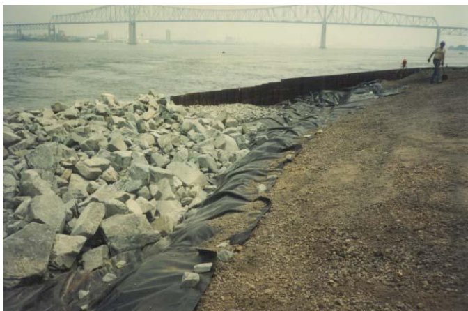
Fig. 15: Failed Area with Lightweight Backfill, Geotextile, Crushed Stone and Riprap
