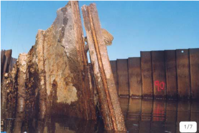
Fig. 10: Brittle Fracture through Interlock
