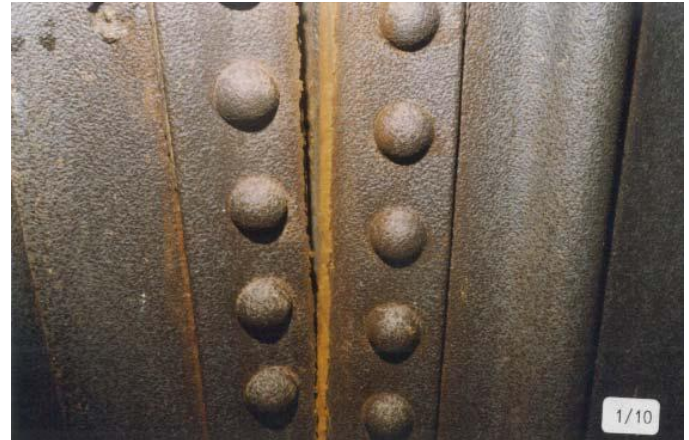
Fig. 11: Connecting Arc A-B in Distress
