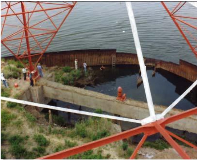
Fig. 5: Partial Collapse Exposing Pile Caps and Tie Beams
