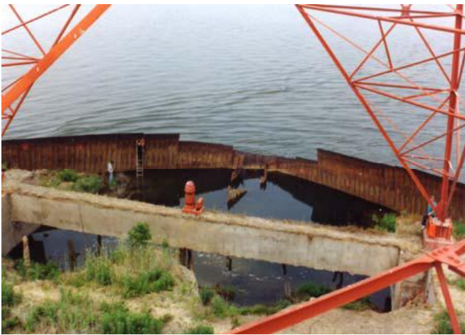
Fig. 6: Partial Collapse Exposing Pile Caps and Tie Beams
