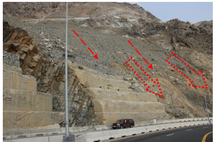
Fig. 9. A debris body include many incised grooves, may fail at the next rainfall incident, where no protection measures are taken.
