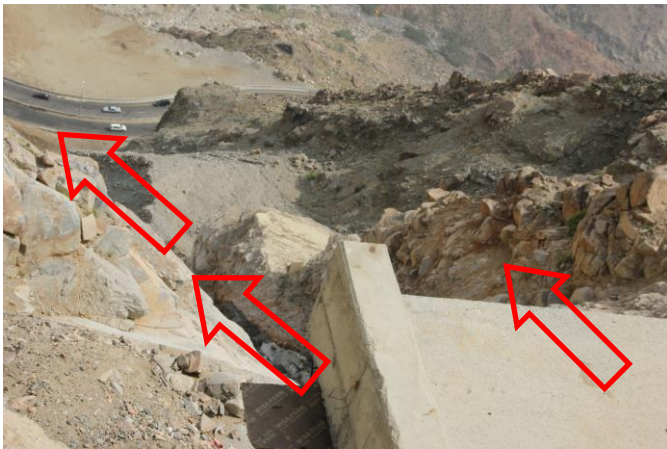
Fig. 8. The presence of the drainage structure directed the drained water to make a path from higher to lower elevations, and ease causing damage in the debris accumulation body below it.
