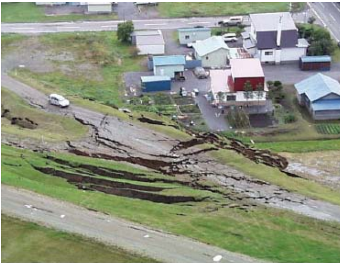
Fig. 6 Damage to embankment at the Tokachi river (After Hokkaido Development Bureau)
