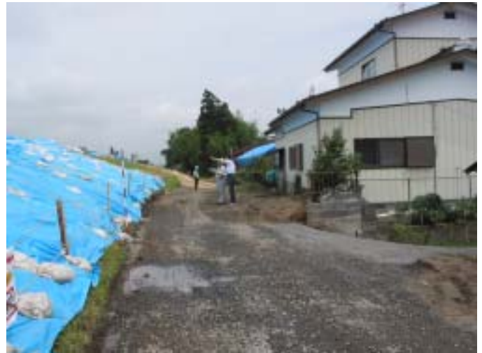
Fig. 5 Residence in the vicinity of the failed river embankment at the Naruse river
