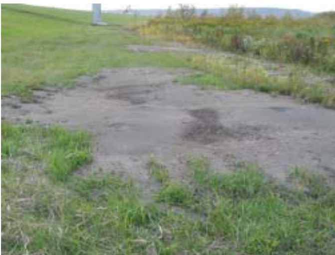
Fig. 7 Sand boils at the toe of an embankment
