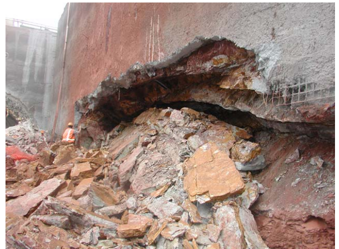
Figure 12: Localized failure along a bedding plane when a double-height bench was excavated.
