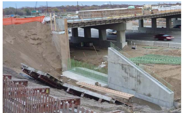
Fig.8. Adjacent retaining wall construction occasionally required the removal of some of the bridge backfill as seen in this photo from November 11, 2011.
