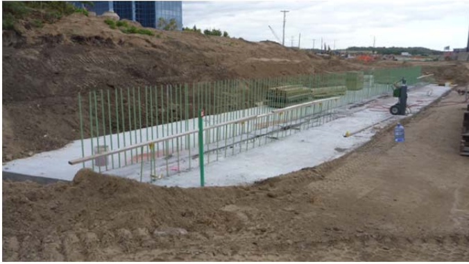
Fig. 5. The footing is cast with an optical target located in the foreground, September 20, 2011.
