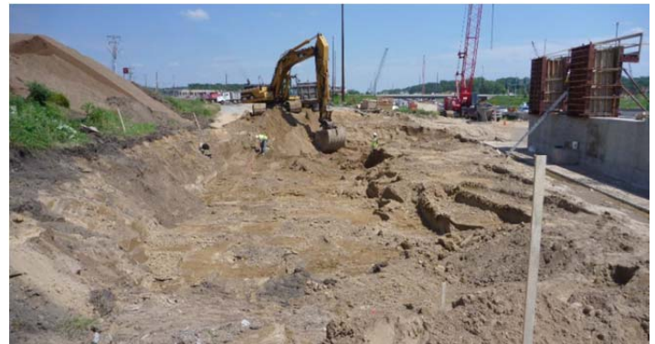
Fig. 3. Excavation of the north abutment area of BR 27R29 prior to placing preload, August 04, 2011.
