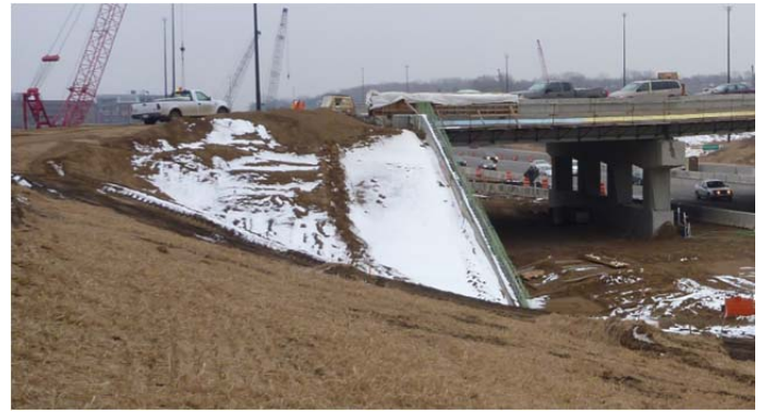
Fig.9. Adjacent retaining walls construction is substantially completed at the North Abutment, November 22, 2011.
