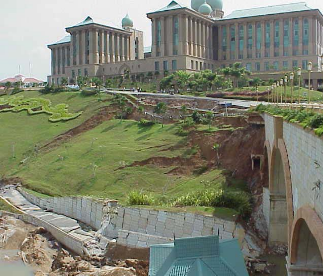
Fig. 2. Extent of the failed area
