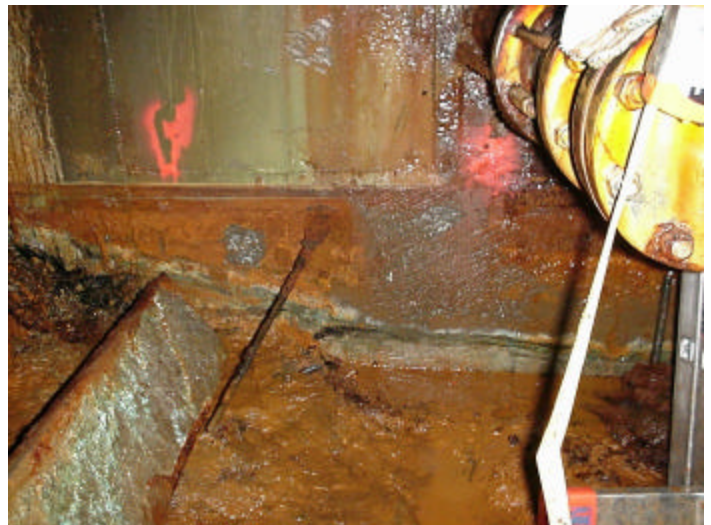
Photo 3. Closeup of bottom left quadrant showing water line of seepage pool (Nov. 2, 2000)
