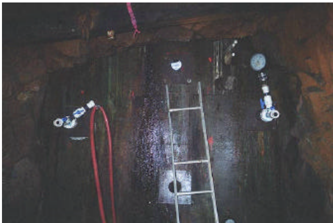
Photo 5. Core holes BH-2, -3, -4 and -7 in the upper half of the seal. Holes BH-2 and BH-4 are equipped with shutoff valves (September 10, 2001).
