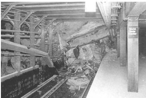
Fig. 8 Damaged subway tunnel.
