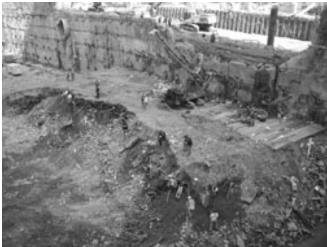
Fig. 15 Section of crushed wall at Greenwich Street
