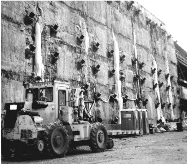
Fig. 14 Icicles form at leaking joints during freezing temperatures
