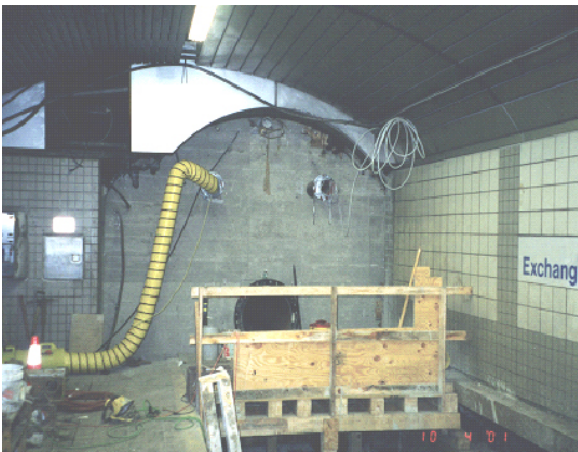
Fig. 7 PATH tube concrete plug.
