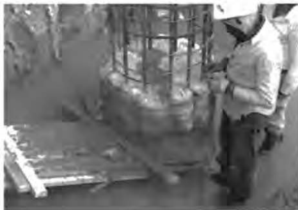
Fig. 11. Grooves in outside surface of caisson
