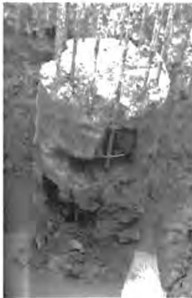
Fig 12. Exposed reinforcing in caisson.
