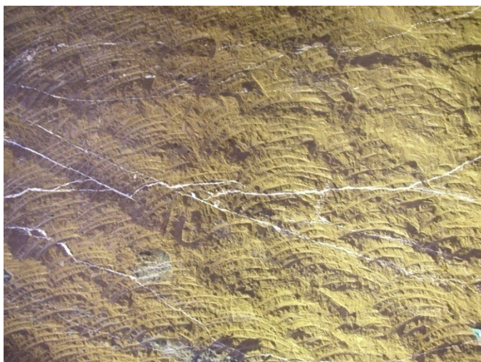
Fig 15. SILACSOL permeation through the cracks system as appeared during the tunnel excavation
