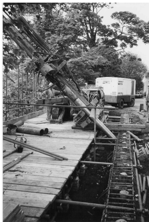
Fig. 7. Anchor installation work from temporary staging (Mini-pile wall capping cage visible in foreground)
