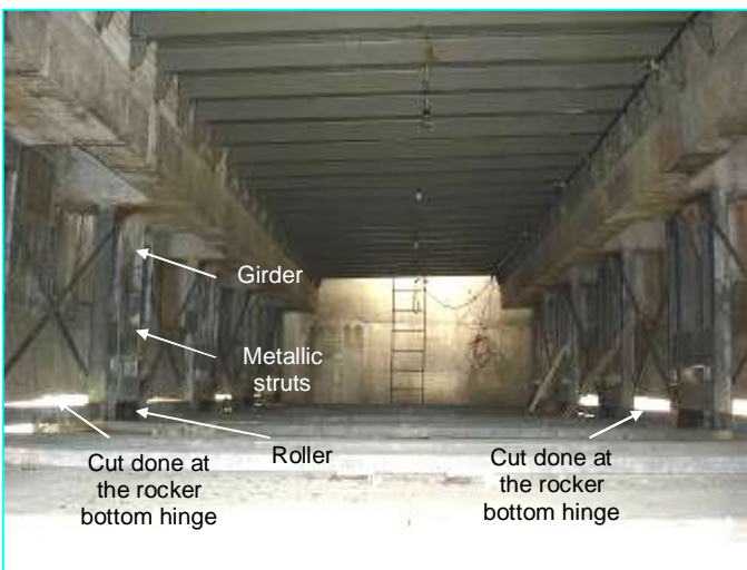
Fig. 17 b Cuts done at the bottom hinge of the concrete rockers located inside the chamber at the Caracas Pilaster
