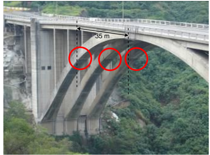
Fig. 23 Location of the fracture at the arch ribs
