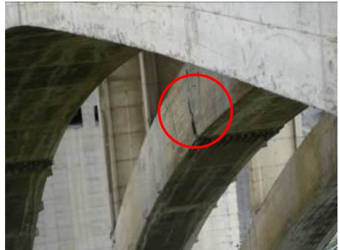
Fig. 24 Fracture of the arch ribs
