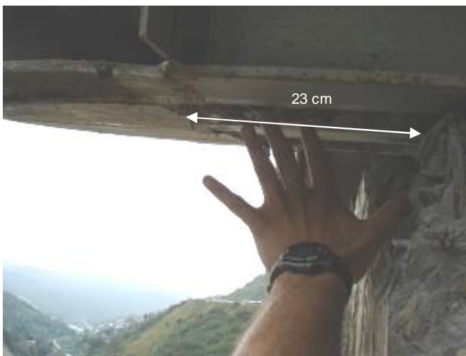
Fig. 18 Transverse displacement recovered at pier 9'
