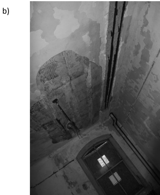
Fig 3. Deteriorated conditions of buildings at the South Island.
