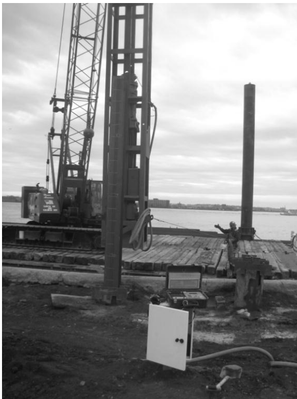
Fig 5. Vibration monitoring enclosing box with Blastmate seismograph.
