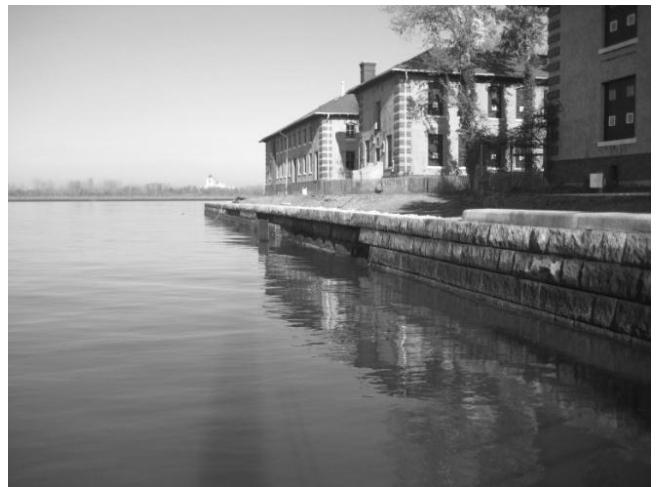
Fig 2. Ellis Island seawalls condition before remedial stabilization.
