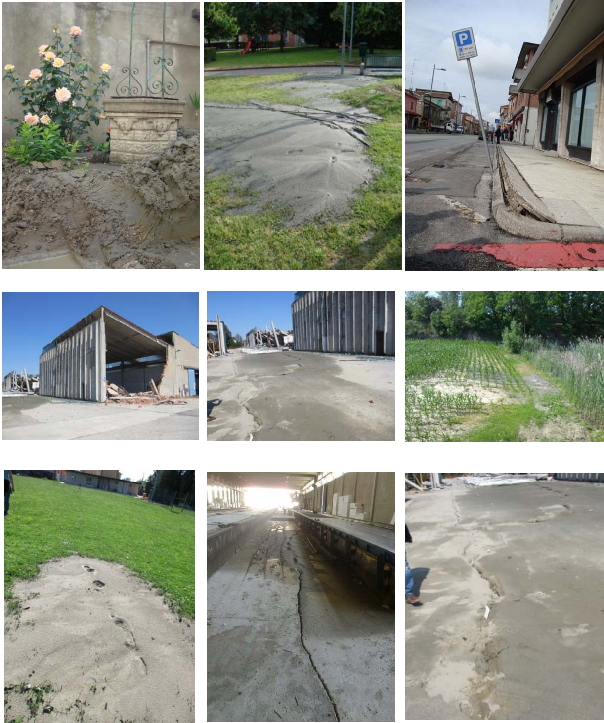
Figure 36. Liquefaction evidences and damages at Mirabello (photos by DICeA Geotechnical team)
