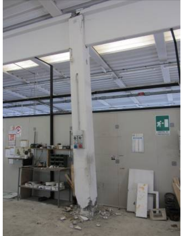
Figure 44. Damage on an industrial building due to hammering on a column by the rigid industrial pavement.
