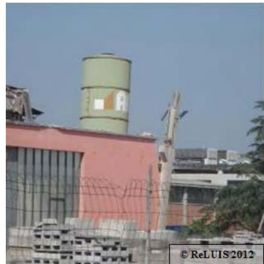
Figure 45. Damage on an industrial building due to foundation rotation.
