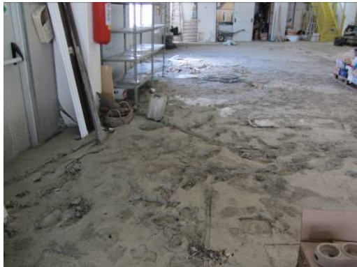
Figure 43. Damage on an industrial building due to soil liquefaction
