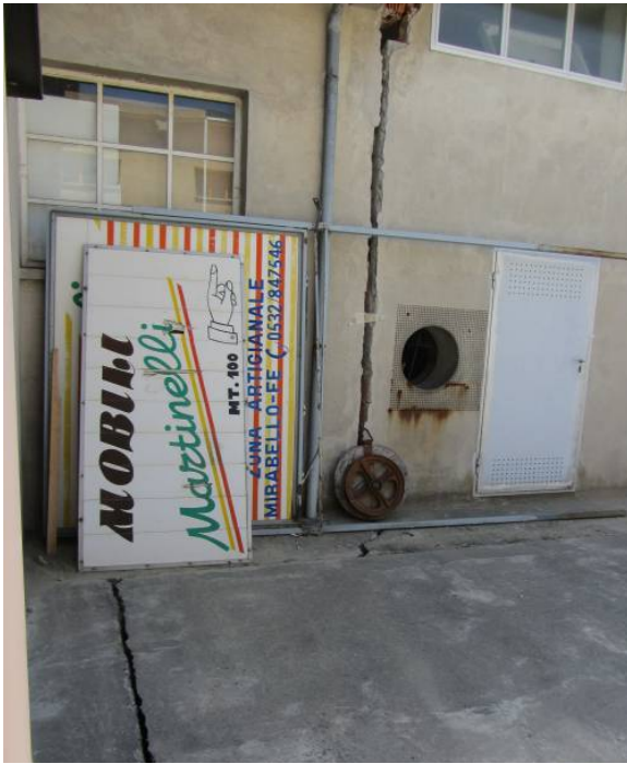
Figure 46. Damage on an industrial building due to fractures in the soil.
