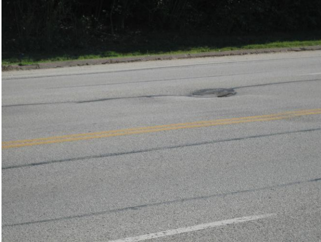
Fig. 15: Sinkhole over leaking sewer.
