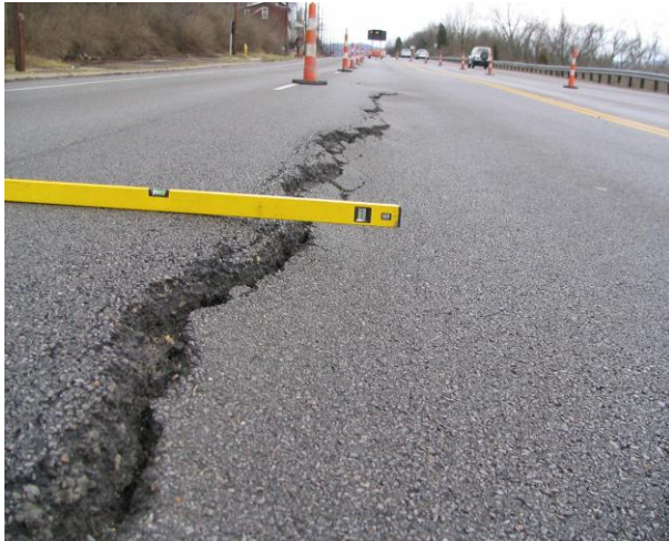
Fig. 2: Road distress and lane closure (2005).
