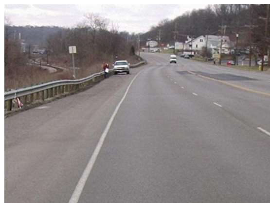
Fig. 1: Pre-repair road distress (2005).
