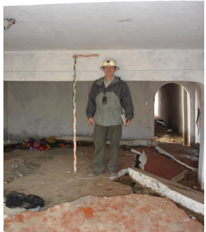
Figure 2b. Interior of a one-story masonry house affected by liquefaction with settlement of approximately 0.7 m. Note the completely damaged concrete slab on ground (GEER 2007)
