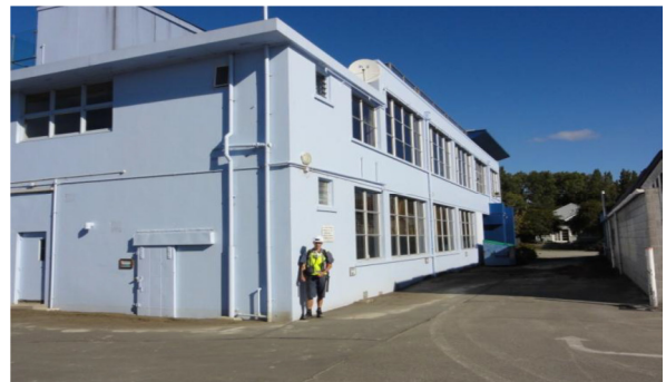
Figure 11. A two-story building subject to liquefaction-induced punching settlements (GEER, 2011)
