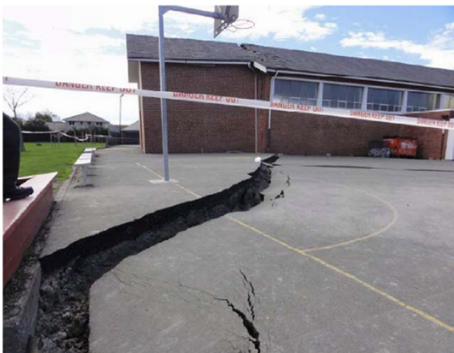
Figure 7. Liquefaction-induced bearing failure at St Paul’s Church (GEER, 2010b)
