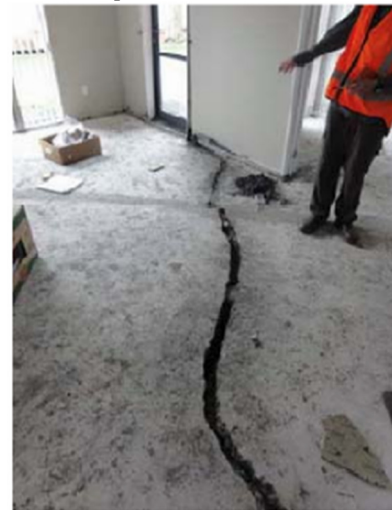
Figure 8b. Cracks in unreinforced slab induced by lateral spreading (GEER, 2010b)
