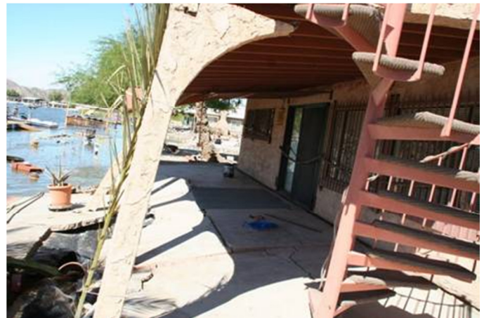
Figure 5 – House affected by lateral spread in Rio Hardy, Baja California, Mexico.
