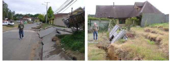
Figure 4. A damaged house located at toe of landslide (left); a damaged house located at head scarp of landslide (right) (GEER, 2010)
