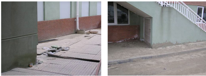
Figure 3 Sediment ejecta observed around Hospital Provincia wings (GEER, 2010)
