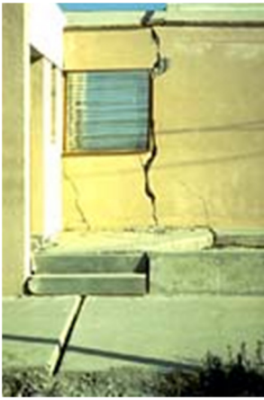
Figure 1a. Liquefaction-induced differential settlement of a one-story masonry house (NISEE 1997)
