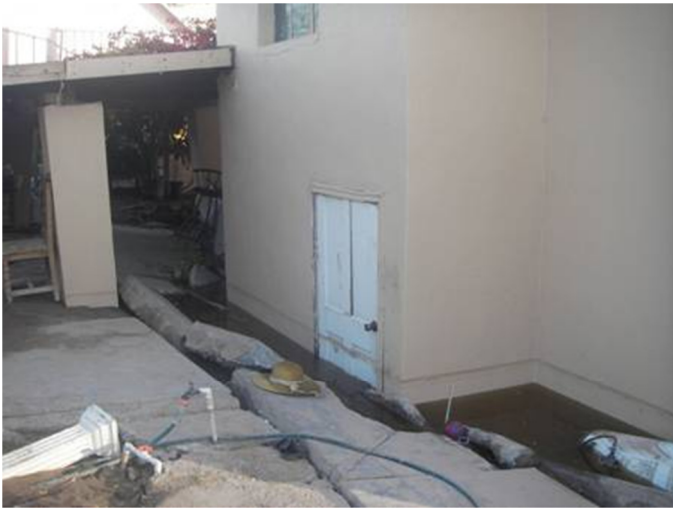
Figure 6 – Settlement of approximately 1 meter in a two-story house in Oaxaca, Mexicali Valley, Baja California.
