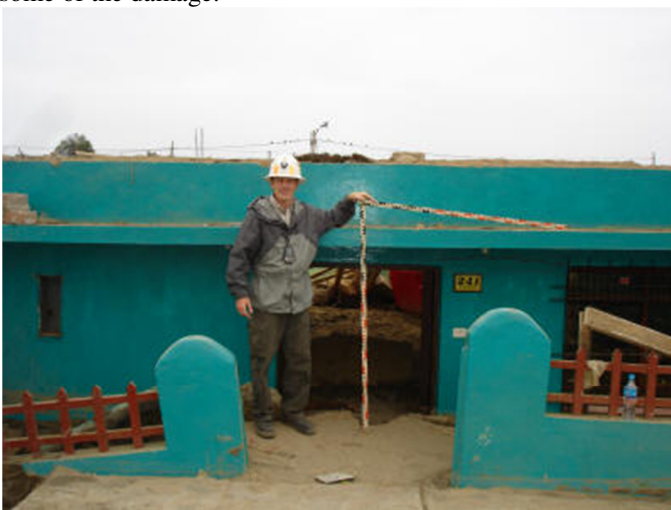
Figure 2a. Liquefaction-induced settlement of about 0.9 m of a one-story masonry house in Tambo de Mora, Peru (GEER 2007)
