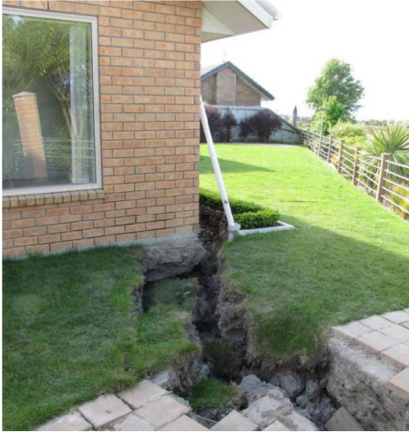
Figure 9. Lateral spreading compromising ground support beneath the concrete slab-on-grade foundation at Kokopu Street (outside of the building) (GEER, 2010b).
