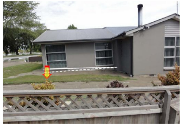
Figure 10. Damage building due to differential settlement (GEER, 2011).
