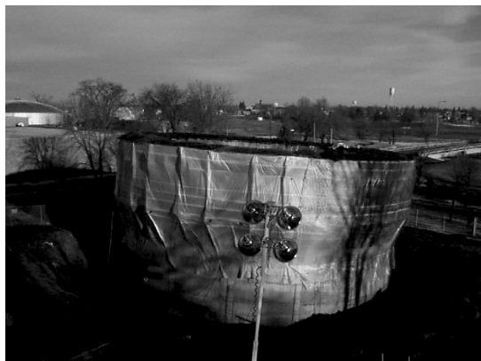
Fig. 5. Photo showing early tilt of caisson
