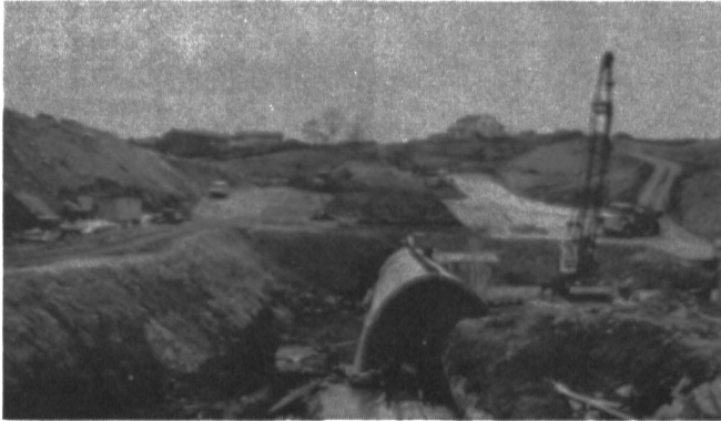
Fig. 7 : Creation of arching at Monistrol-sur-Loire (Haute-Loire)
