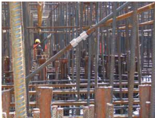
Fig.13. Layout of field steel bar sensor on downstream cap of 4# pier
